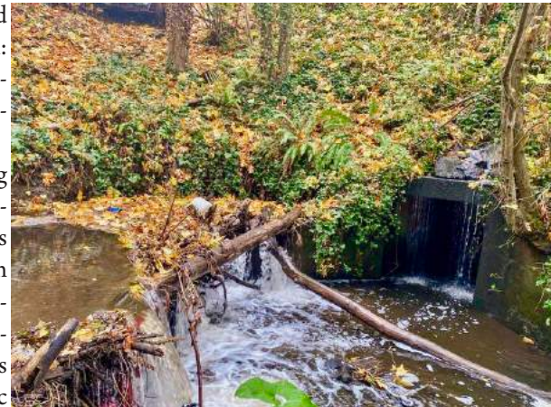
A culvert in Seattle's Lake City neighborhood, rated 67% passable for salmon. (Ashlee Abrantes/CC BY-ND)
